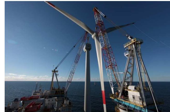
Alpha Ventus Offshore Wind Farm 1
